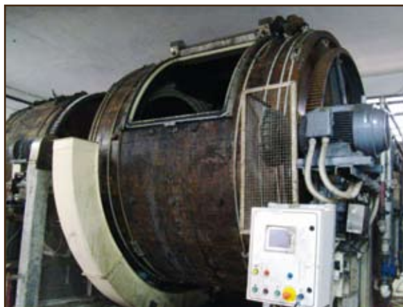
1. reparto bottali - drums area
