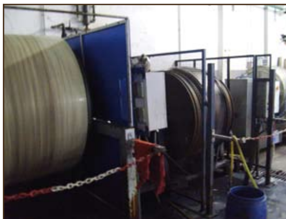
2. reparto bottali - drums area
